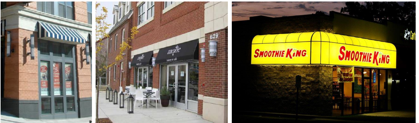
Left: awning installed too high; Center: Awning not deep enough; Right: Backlit awnings are not allowed
